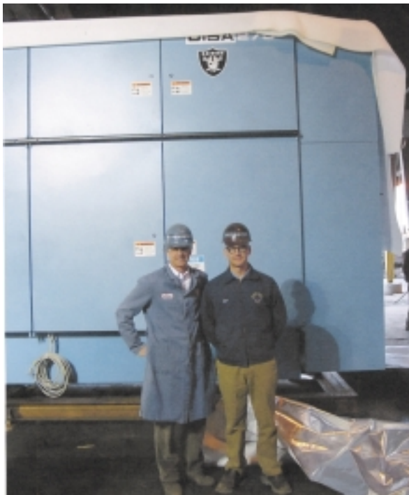
AB&I president, Allan Boscacci, and Chief Operations Officer, Kurt Winter, inspect the new Disa 270 during its recent installation.
