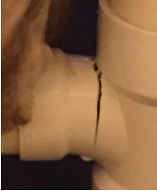
Figure 3: Cracked PVC fitting (Picture by James A. Richardson Jr.)
